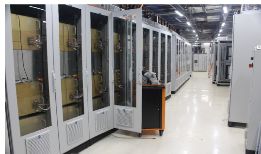
Figure 9: Sirius power supply room, with booster dipole PS at the forefront.
