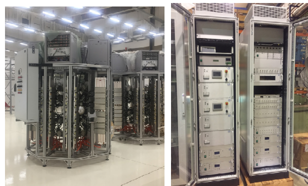
Figure 8: Storage Ring 60 kW SSA stored in the RF room on the left, and interlock and LLRF systems in the RF lab waiting for installation on the right.
