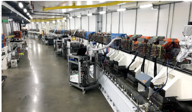
Figure 3: Accelerators tunnel with the completed booster installation (inner accelerator) and a storage ring sector being assembled.
