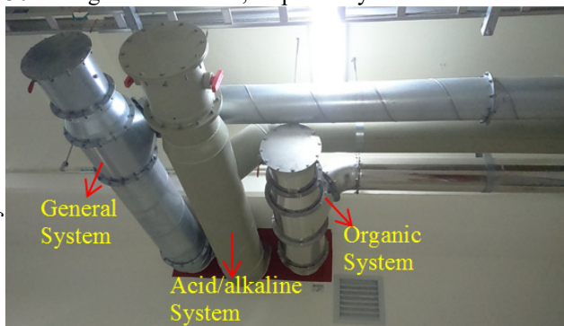
Figure 3: Typical ducts layout of three laboratory exhaust gas treatment systems in a laboratory in the TPS.
