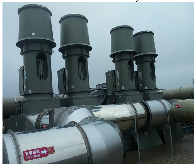
Figure 1: Four fans of the Acid/Alkaline and Organic systems.
