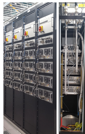
Figure 8: (LEFT) RF amplifier racks in LS1. (RIGHT) Rear view of 2 x 4 kW amplifier rack (80.5 MHz).
