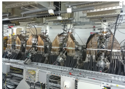
Figure 2: RF Cavities Section.
