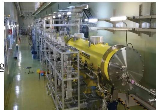
Waveguide system completed (just recently)
