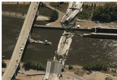
Figure 1: Fall of aged bridge accident in America [3].
