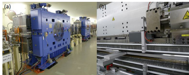
Figure 1: (a) Installation of two EPU48 in the TPS storage ring. (b) Protection of a linear encoder with a lead shielding box.
