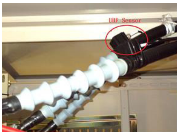
Figure 7: One of UHF sensors installed at the cable termination of 22.8 kV transformer.
