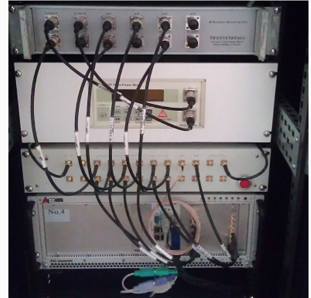
One typical control unit
