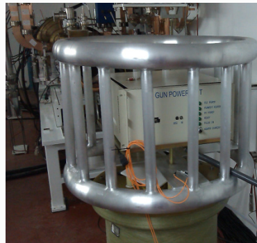
HV station (150kV Max)
