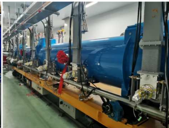
Cryomodule in tunnel
