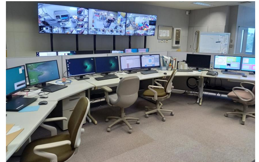
Figure 6: NewSUBARU control room
