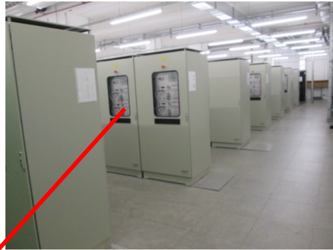
Main Power Supply Room
