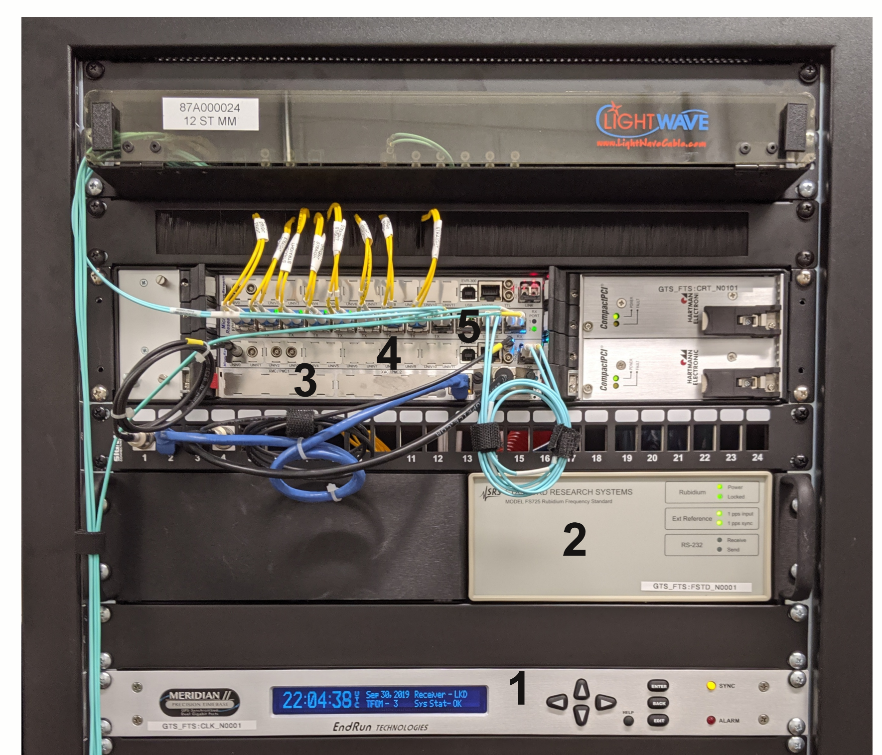
Figure 7: Timing master hardware. 1) GPS/PTP/NTP grandmaster, 2) 1 PPS/10MHz Rb oscillator, 3) cPCI CPU card running real-time Linux kernel, 4) Master event generator with 1 PPS and 80.5MHz inputs, 5) Fan-out distribution to facility; yellow cables are 10Gb/s single-mode fiber, cyan cables are 1Gb/s multi-mode.
