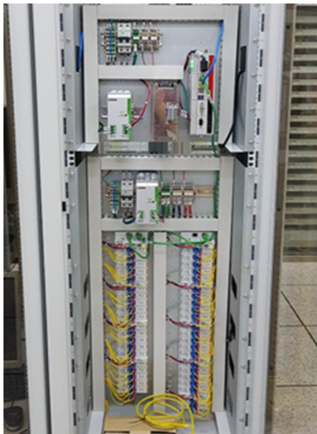
Figure 4: EtherCat Master unit in Server Room Rack.
