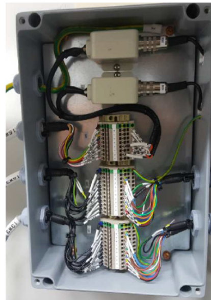
Figure 2: Junction Box in tunnel wall.
