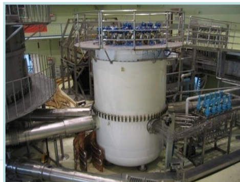
Cryogenic distribution system
