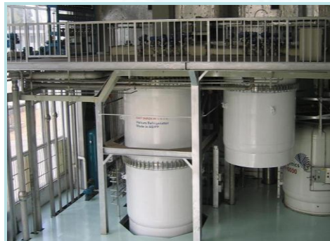
2kW/4.5K Helium Refrigerator
