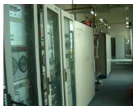
RF Power Supply System (use PLC Controller)
