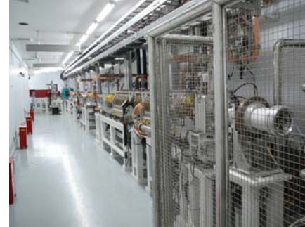
150 MeV Linear accelerator tunnel
