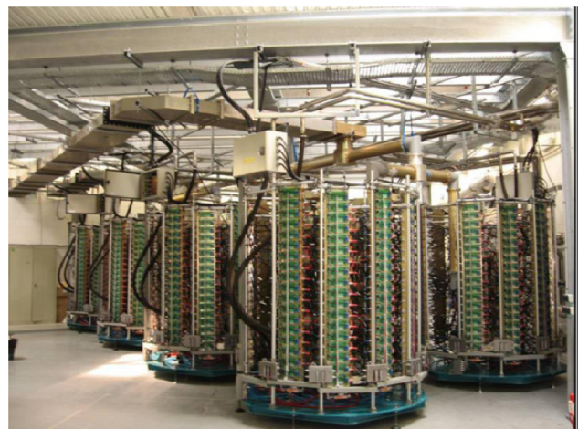
Figure 7: Solid state RF amplifier at Soleil.
