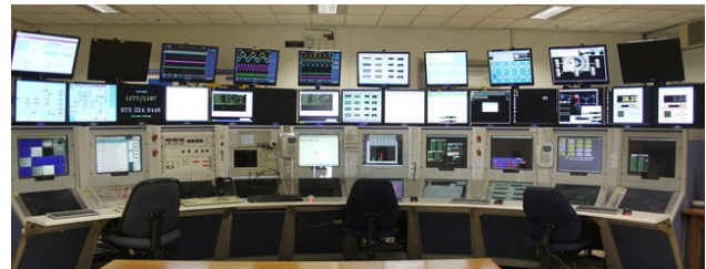
Figure 2: The renovated Control Desk.
