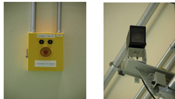
Figure 3: Emergency stop button & Monitoring camera.
