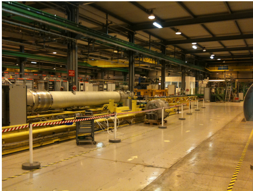
Figure 1: Part of the merged MTB facility.
