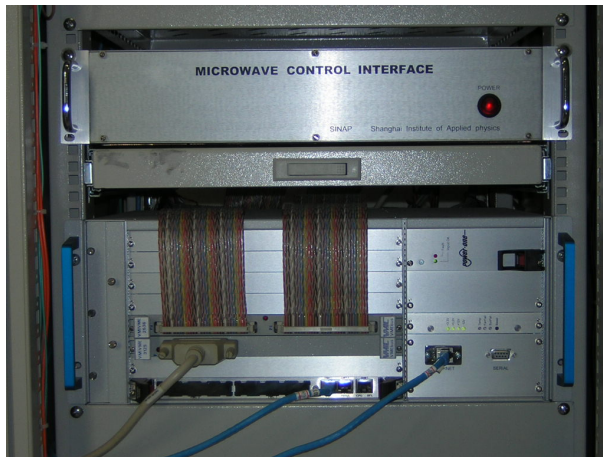
Figure 4: IOC controller and Interface.
