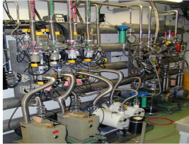
Figure 9: Exhaust gas collecting station.
