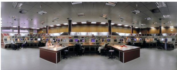
Figure 7: Main Control Room at GSI.
