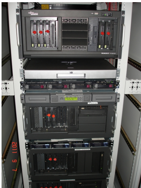
Figure 3: One of the ACS 19'' racks.
