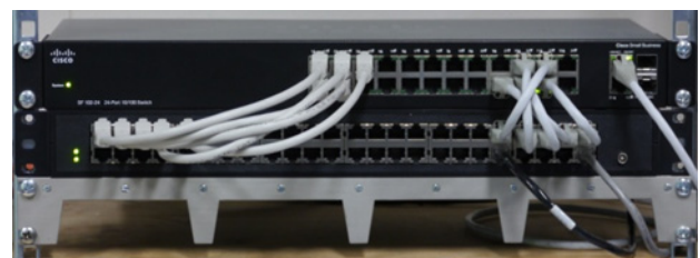
Figure 6: Ethernet switch and sync pulse injector.
