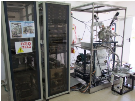
Figure 2: LiLiT target and control racks in the off-line lab
