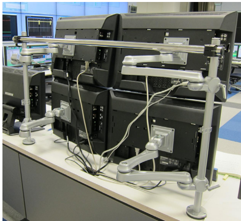
Figure 4: A desk has two poles to support 4 LCD panels.
