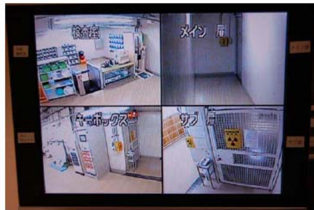
TV Monitors of an Access Point
