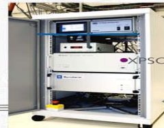
Rack with device controllers
