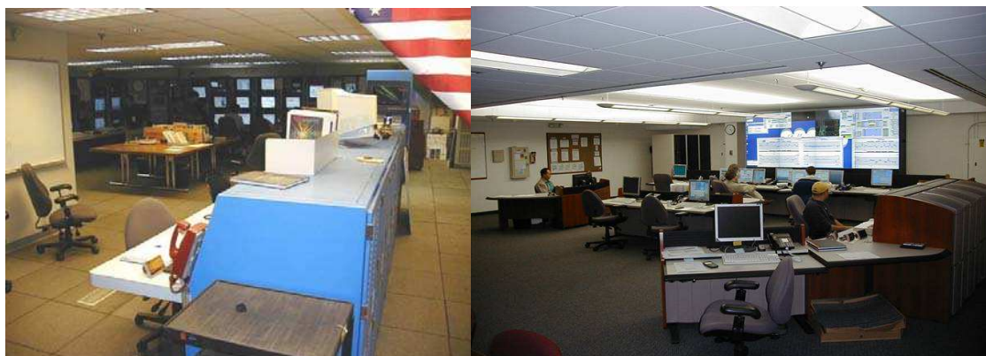
Figure 1: Old control room (left) vs new control room
