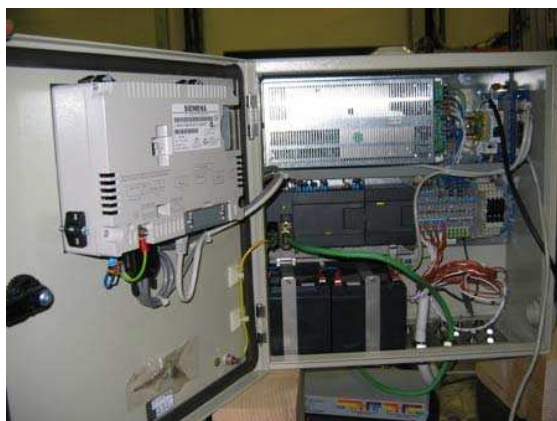
Picture 1. Inside the control unit of a monitoring station.
