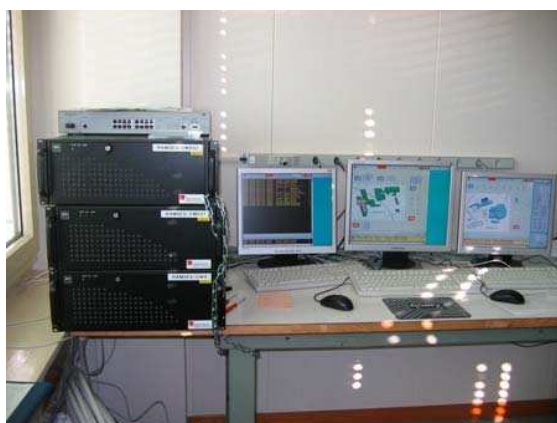
Picture 3. Central supervision: redundant servers and screens.
