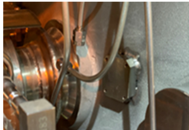
Figure 3: Picture of the welded detector holder on the dipole endcap.
