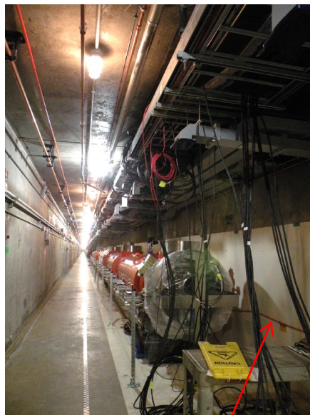
LBLM A-chain fiber: On north wall at beam height, 90 cm from beam
