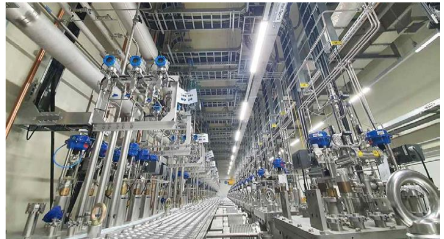
Cryogenic Distribution to Cryomodule
