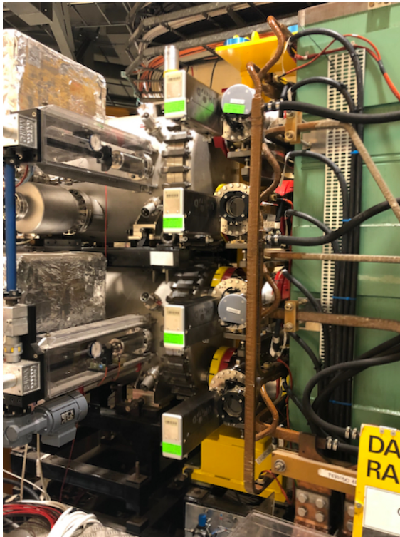
Figure 3: Four BTVs installed in the PSB.
