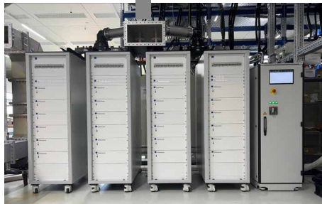
SSPA Rack system powering the accelerator
