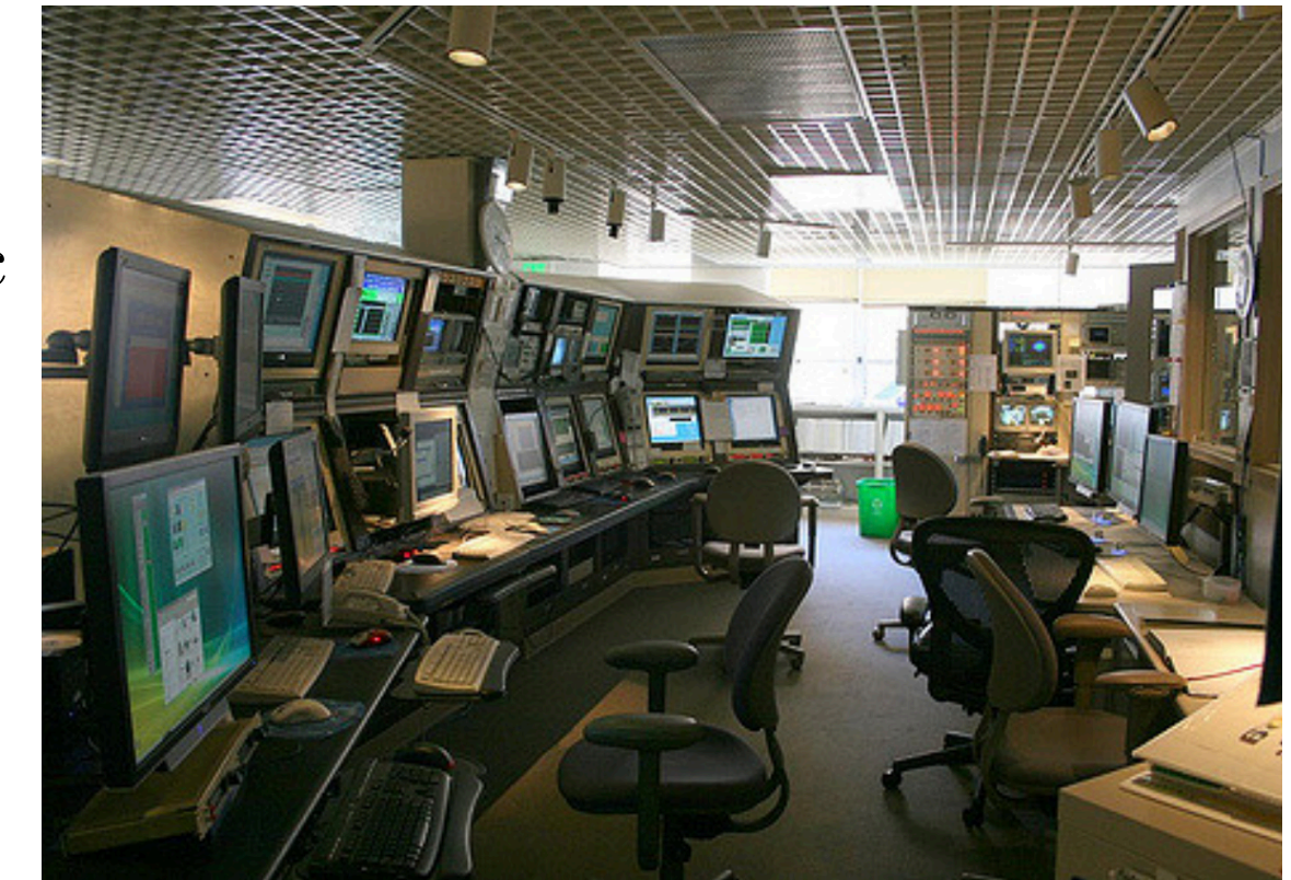
High level controls
