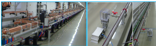
Figure 4: Condition of installed waterpipes and HLSs (Linac on the left and Undulator on the right).
