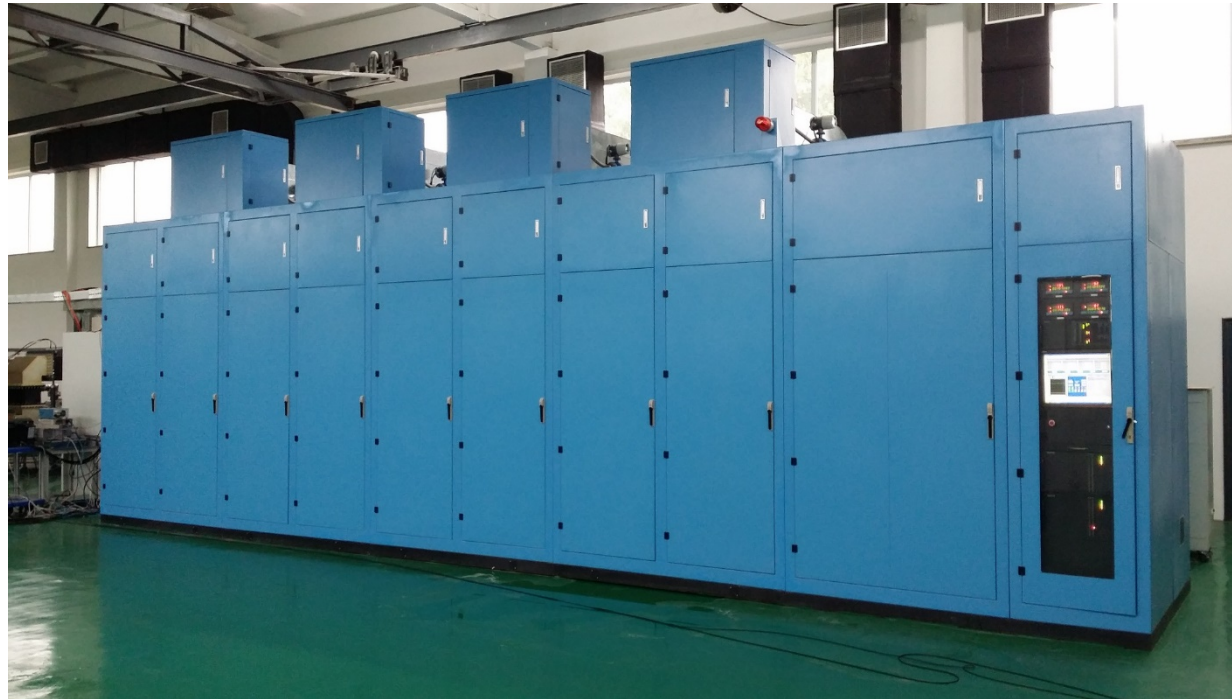
ADS 80kV/18A PSM Power Supply
