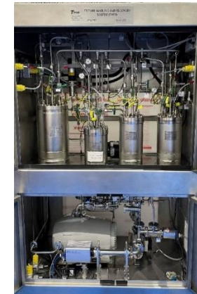
Tritium Handling and Recovery System
