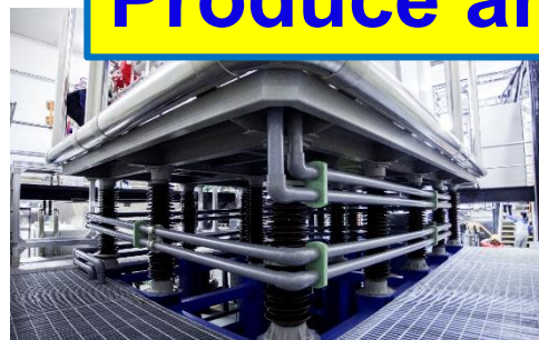
High voltage platform
