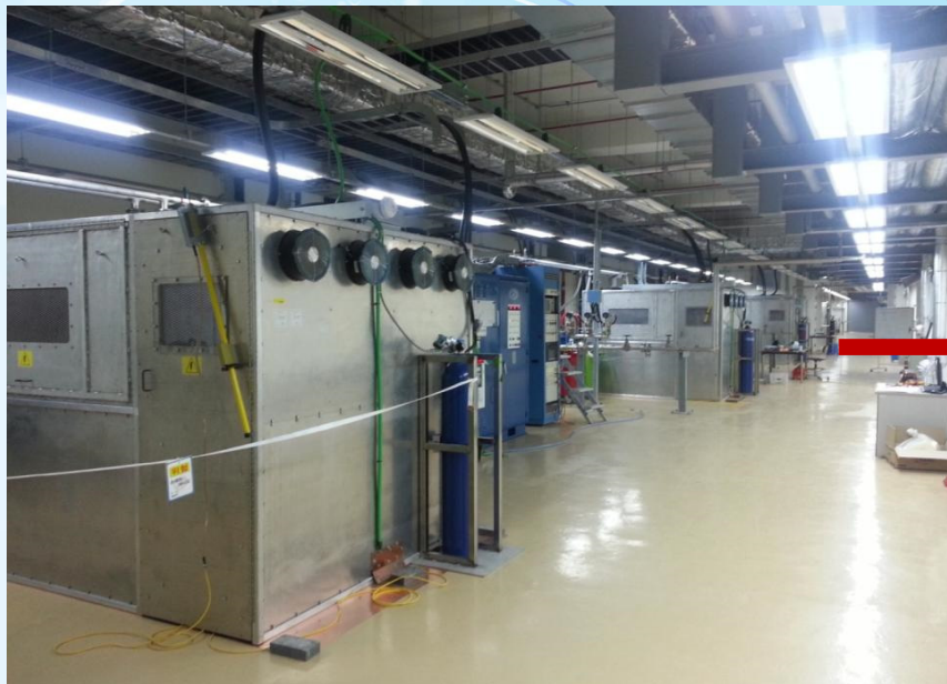
Modulators on 3 rd floor
