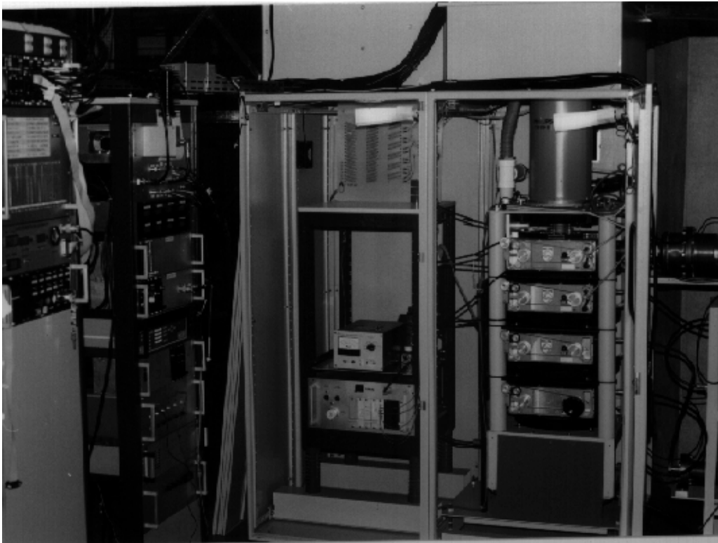
Figure 2: RF amplifier and control panels.
