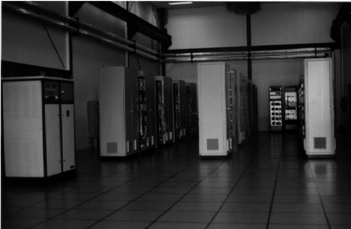
Figure 1: power supply room of the LNLS.
