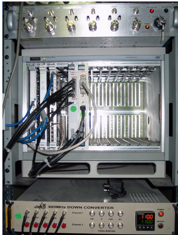
Figure 1: LLRF Control System
