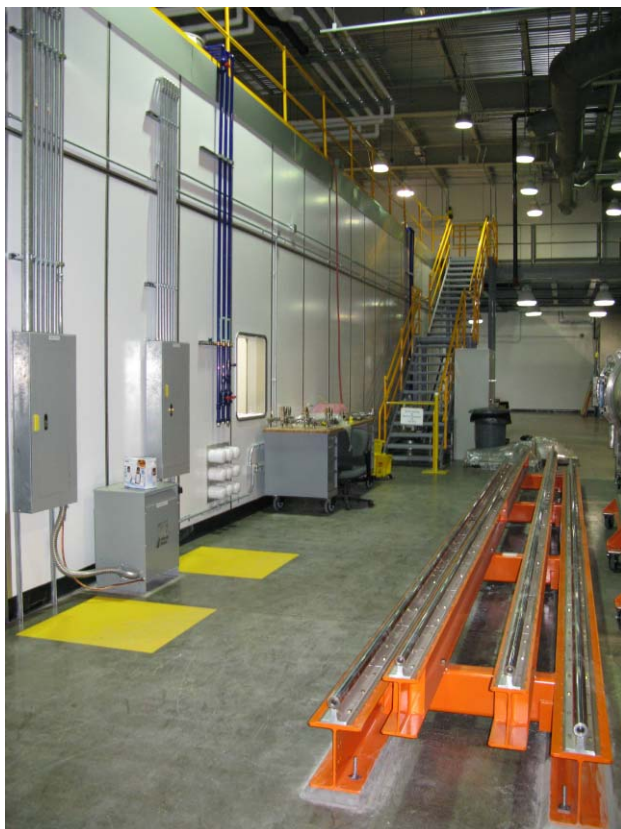
Figure 2: Exterior view of Cleanroom and Cryomodule Assembly Rail
