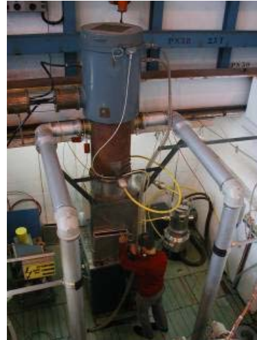
Figure 5: The 2 MW amplifier; in the right corner its driver is visible.
