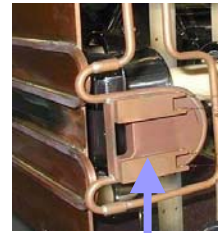
Beam-loss diagnostic inside cyclotron
