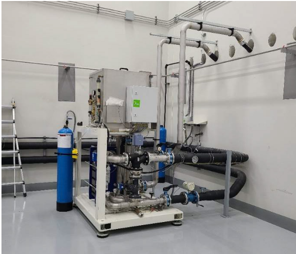
Cyclotron cooling room
