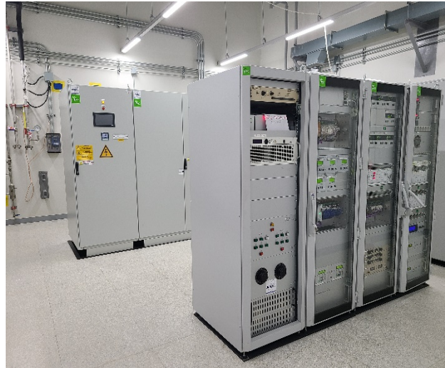
Power Supply room
