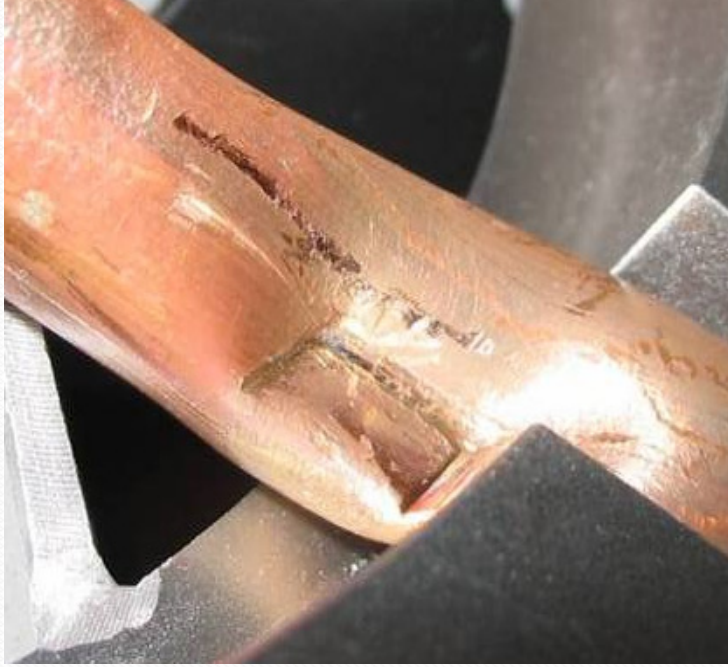
Corroded pipe cooling
