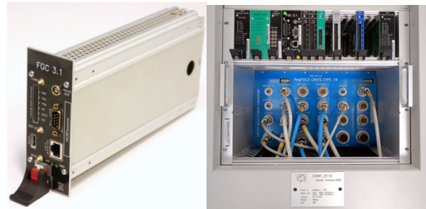
Figure 3: FGC3 controller and Type-10 RegFGC3 Crate.
