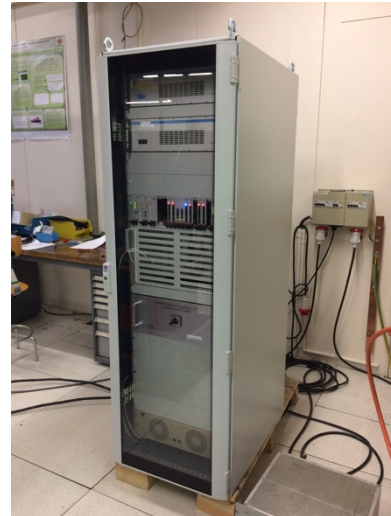
Figure 5: Air-conditioned cabinet for the DCCT and controls electronics.
