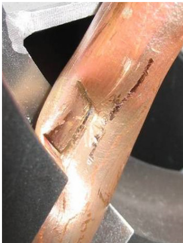
Figure 4: an example of corroded pipe cooling.
