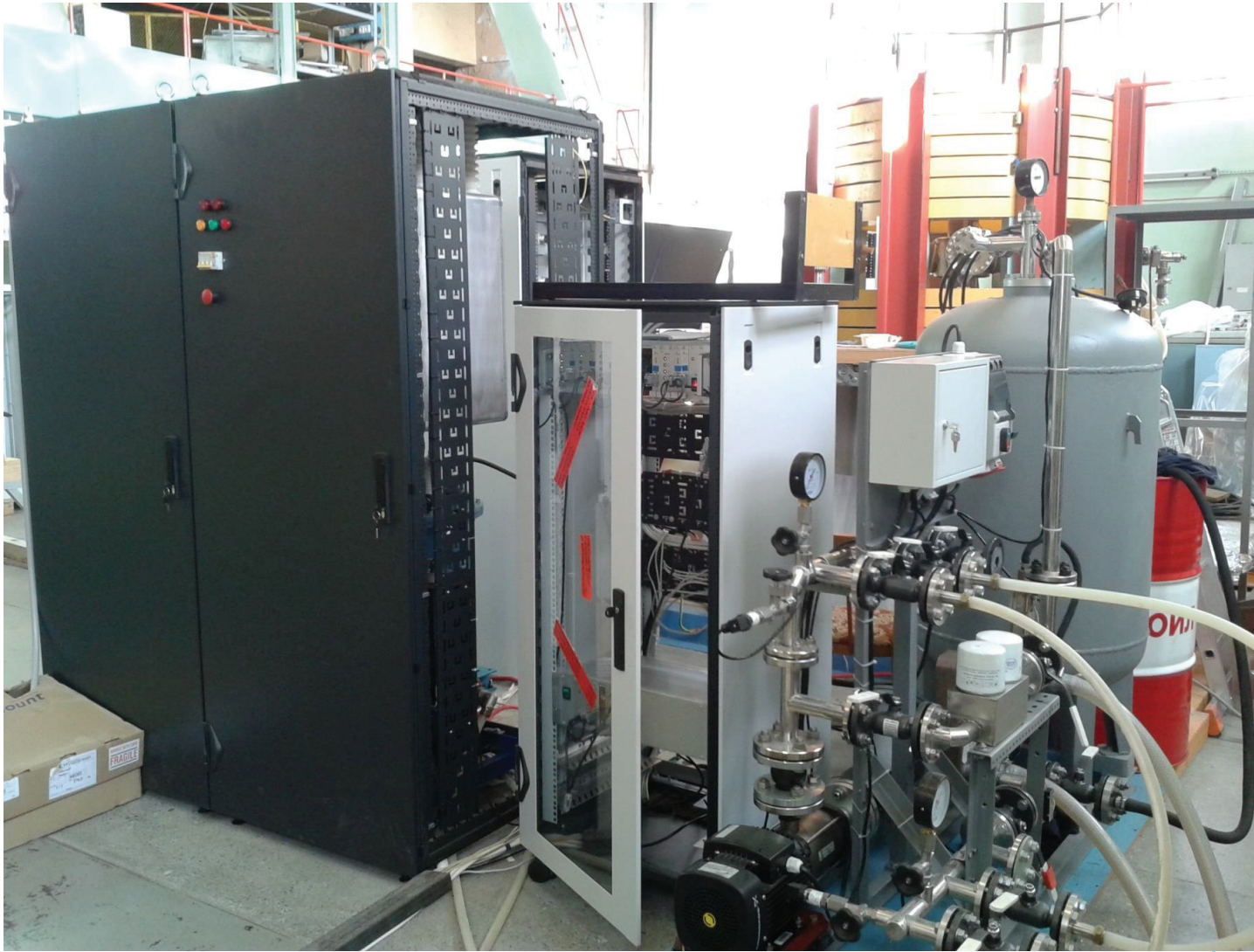
60 kV power supply and oil cooling system
