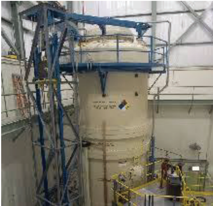
FNAL 4.3 MV TEVATRON cooler 2005
