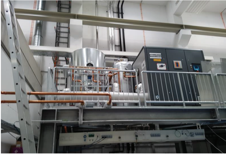
Compressor station for up to three turbines
