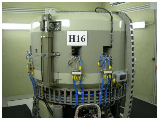
Figure 1: IBA CYCLONE 18/9 – H16 inside the bunker
