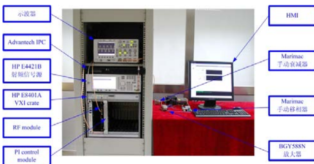
Figure 14: The digital low level RF control system
