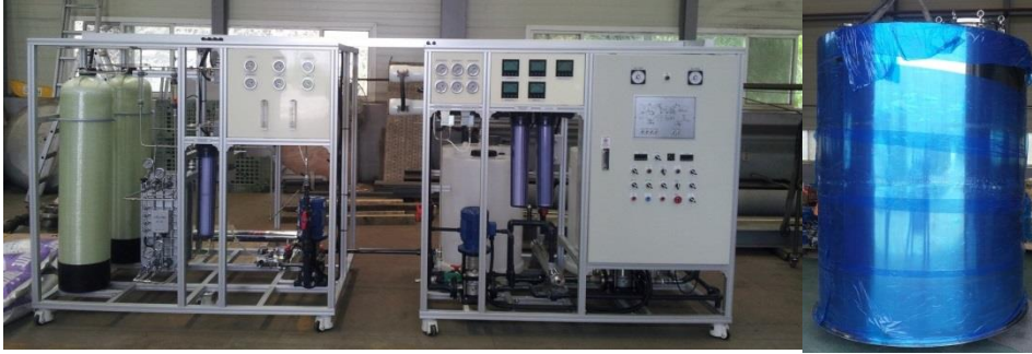
DI water system (completed)
